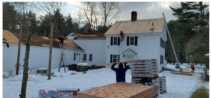
Photos above: two views of the start of our new roof at Squire's Tavern (January 25, 2022). The job was finished a couple of days later—thank you to our contractor: Royal Construction (Canton, CT 860 693-2806).
